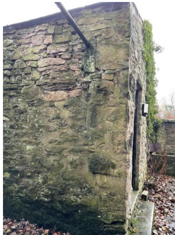
(25) Poor quality rubble walling
