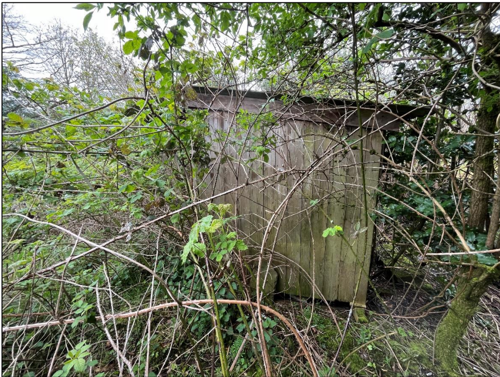
Plate 4 – Overgrown and dilapidated nature of B3
