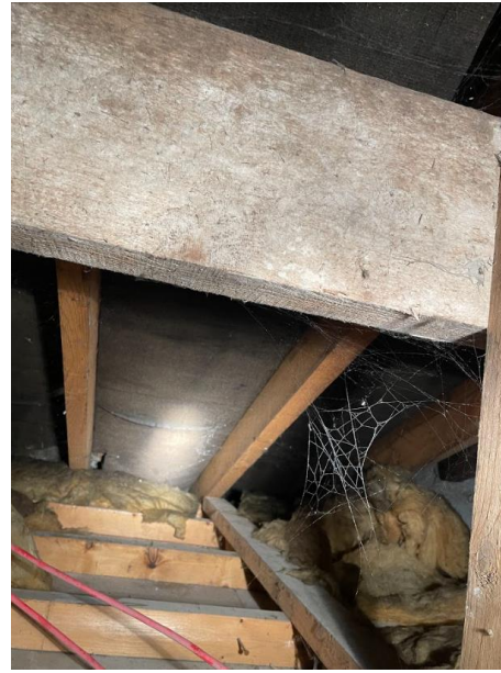
Photograph 6 – First floor loft void with tear in insulation fabric present
