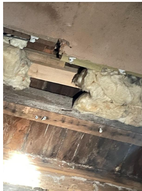
Photograph 12 – Damage to the underpass roof exposing gaps in the insulation material
