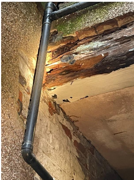
Photograph 11 – Rotting wood exposing crevices within the underpass
