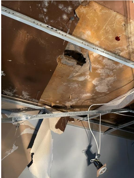
Photograph 1 – Damaged false ceiling
