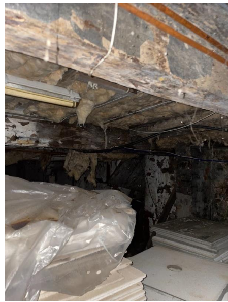
Photograph 4 – Damage within cellar
