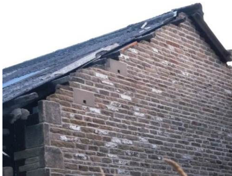
Example of Forticrete boxes in situ
